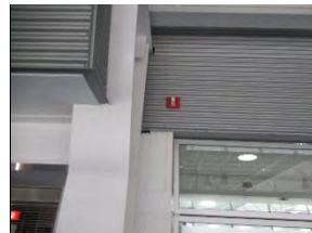
17 WMC 2nd Floor Arena visual alarm
