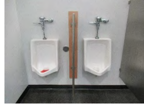
10 MCC Mens washroom urinal area
