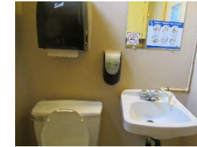
13 SJL Lower level staff washroom sink area
