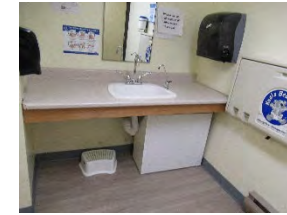
6 EL - Universal washroom sink area
