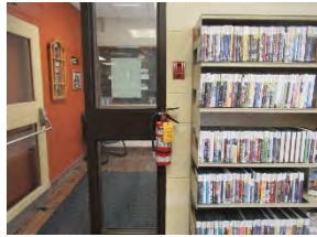
2 EL - fire pull and extinguisher
