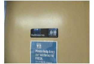
7 SJL - lower level washroom door - no accessible signage
