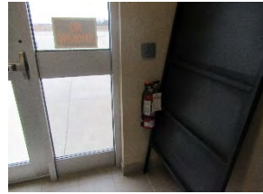
3 FFS - fire extinguisher
