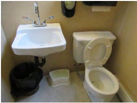
8 SJL - lower level washroom toilet and sink
