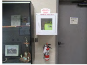
4 BCC Defibrillator and fire extinguisher
