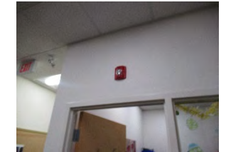
14 WAO office area - visual alarm
