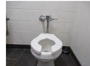
20 WAO Basement - unisex washroom - no grab bars
