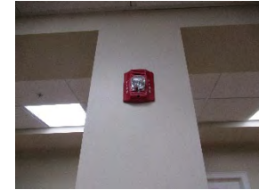
13 BCC Visual alarm installed
