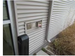
4 BFS - entrance controls
