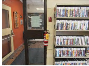
2 EL - fire pull and extinguisher
