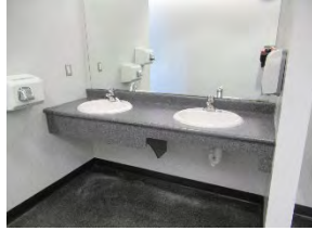
9 MCC Mens Washroom sink area
