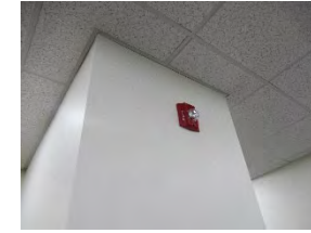
27 WAO 2nd floor - visual alarms
