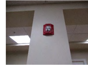
13 BCC Visual alarm installed
