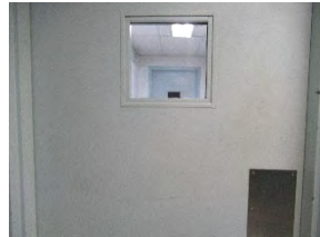
11 SJFS - Door to Mens Locker room no signage
