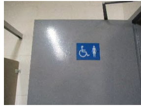
2 SJA - Womens washroom signage
