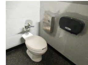
20 SJA - Change room 6 toilet stall
