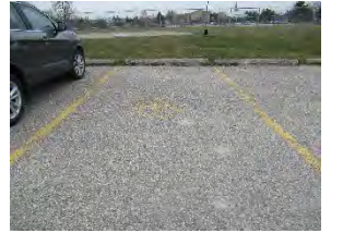
7 ELPW accessible parking
