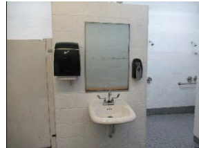
10 WMC Team room 4 - sink area
