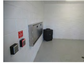
4 GP Universal washroom 1 - controls
