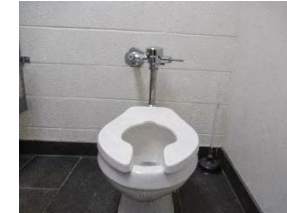
20 WAO Basement - unisex washroom - no grab bars
