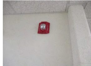
17 WAO Basement washroom visual alarm on outside of washroom
