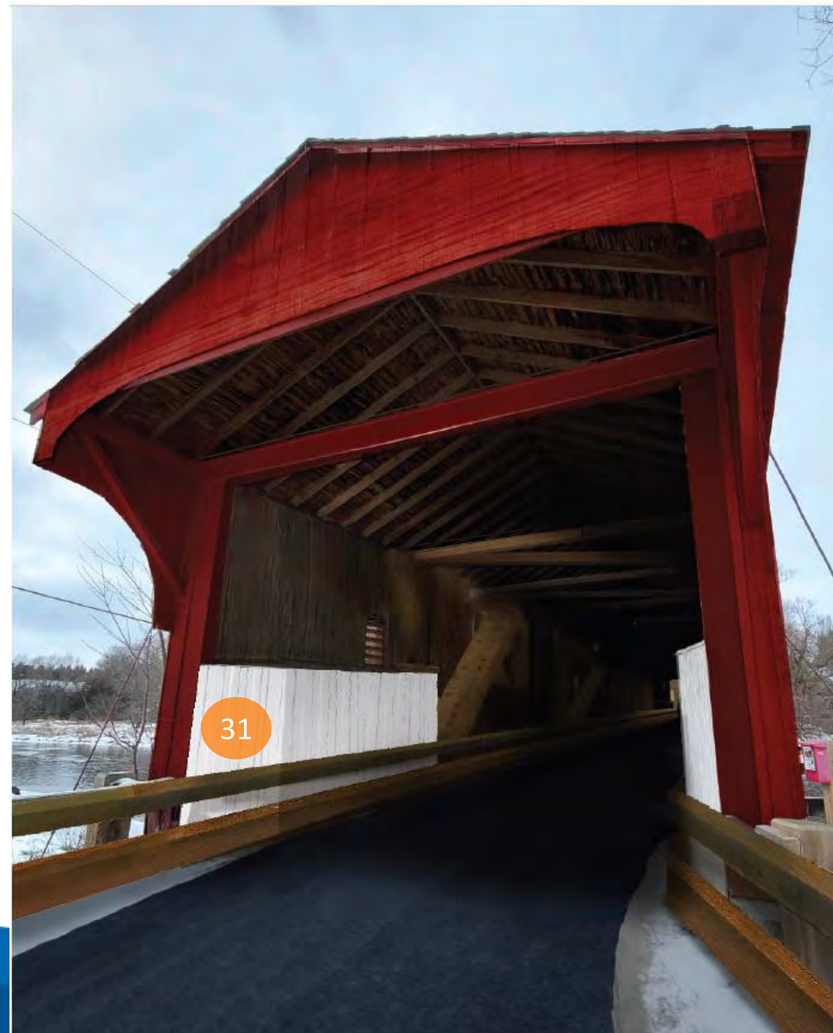
31 Reinstate interior cladding in short sections at each end of the bridge
