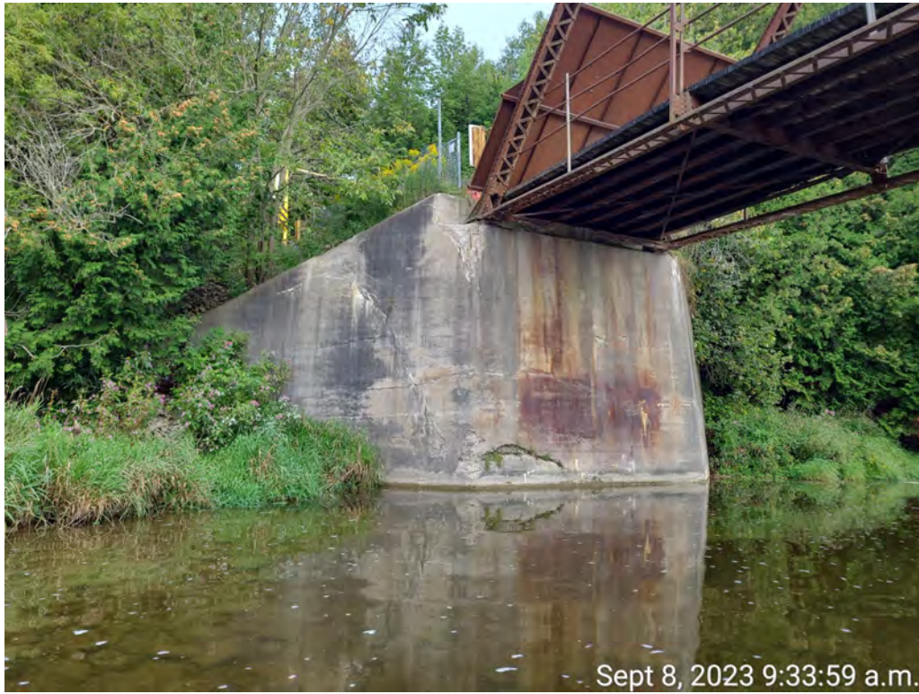
Photograph 15: West abutment showing light to severe erosion, spalling and disintegration.
