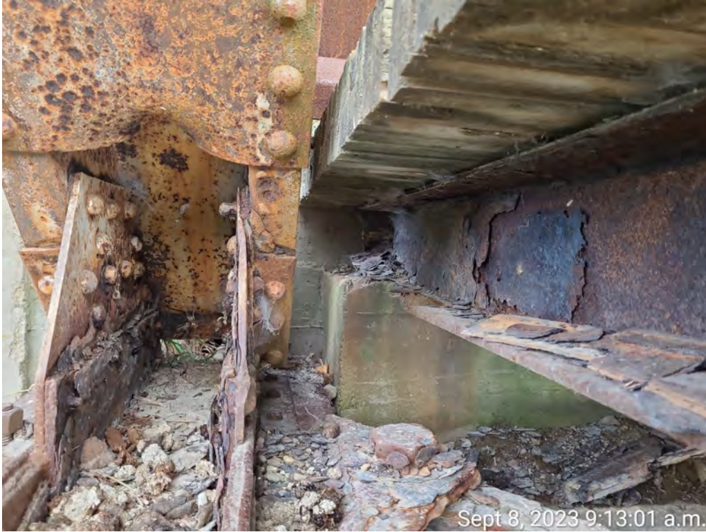
Photograph 3: Stringer in Bay 9 and west abutment, south bearing. Note complete loss of section in stringer bottom flange at stringer bearing seat, severe corrosion of bearing plates and severe corrosion of bottom lateral.
