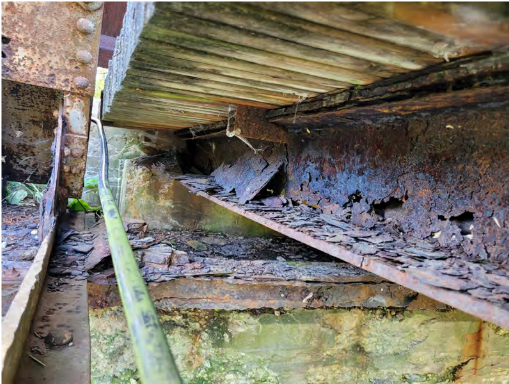
Photograph 5: Stringer in Bay 1 and east abutment, north bearing. Note complete loss of section in stringer web, corrosion in stringer top flange, severe corrosion of bottom lateral and loss of section of stringer flange at stringer bearing seat.
