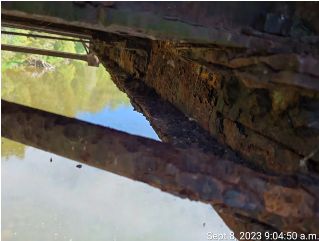
Photograph 8: Bay 8, east end showing severe corrosion of bottom lateral and floor beam.
