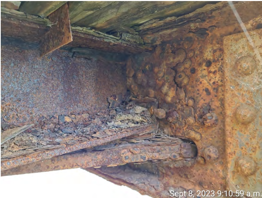
Photograph 6: Bay 9 stringer at east end showing bearing support angle severe corrosion, severe corrosion of floor beam and severe corrosion of bottom lateral.
