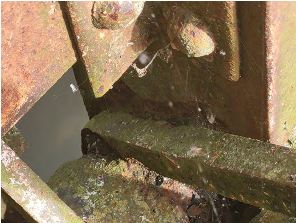
Photograph 12: North truss, Joint 4 showing section loss at diagonal eye bar and vertical web plate.
