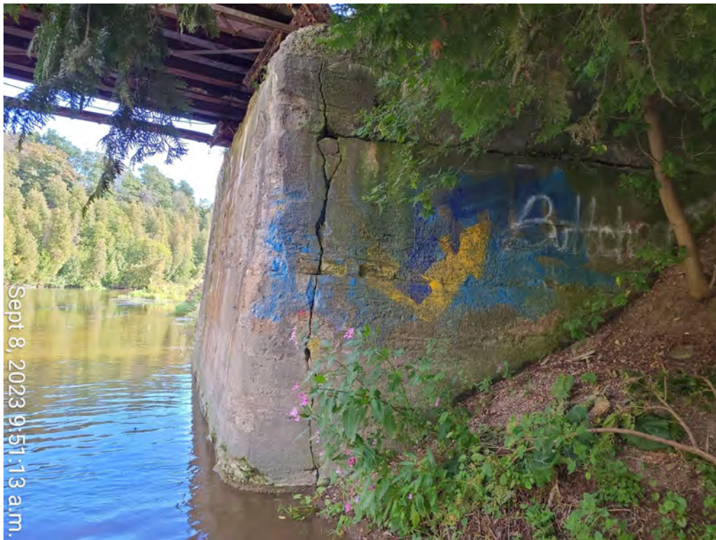
Photograph 17: East abutment, south wingwall showing wide vertical crack at wingwall/abutment interface and wide horizontal crack at cold joint.
