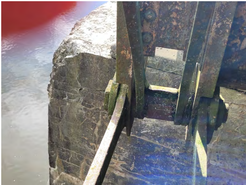
Photograph 10: North truss, Joint 6 showing light to severe corrosion of eye bars and vertical web plates as well as crack in bottom exterior chord.
