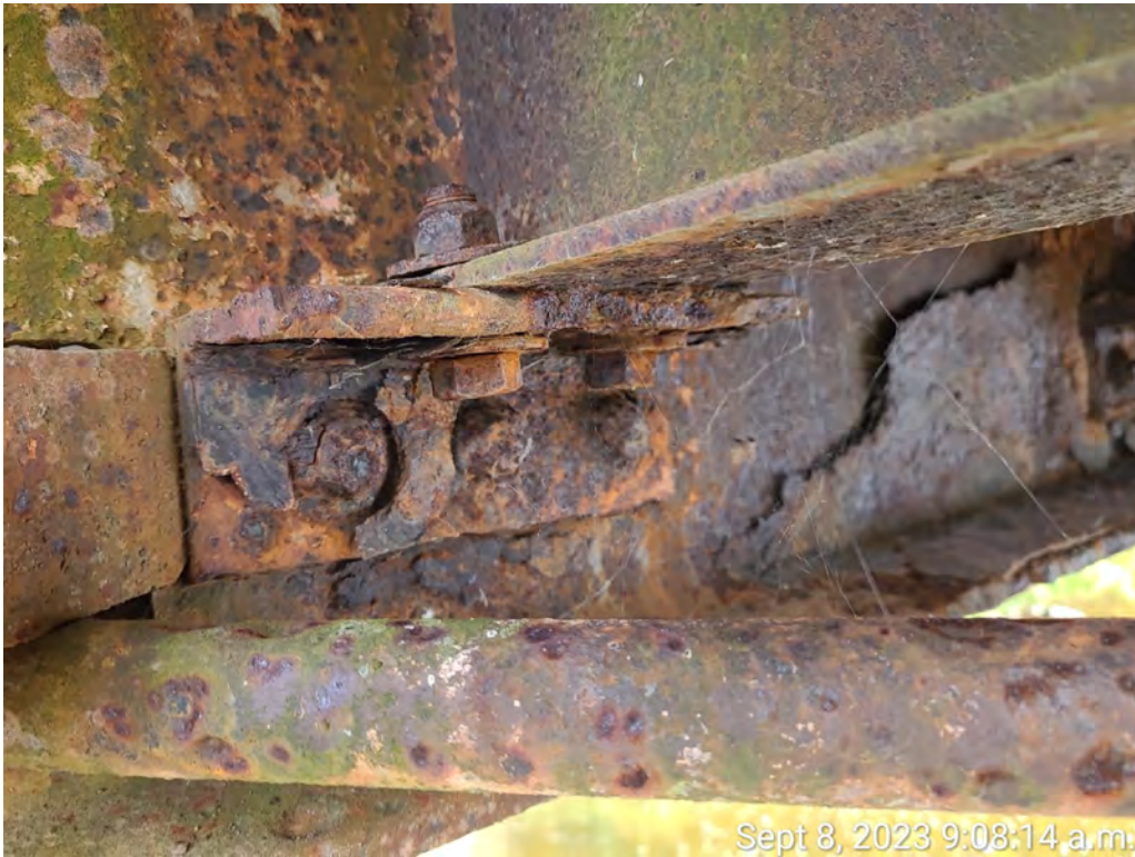
Photograph 7: Bay 8 stringer at west end showing severe corrosion of floor beam and severe corrosion of stringer bearing support angle.
