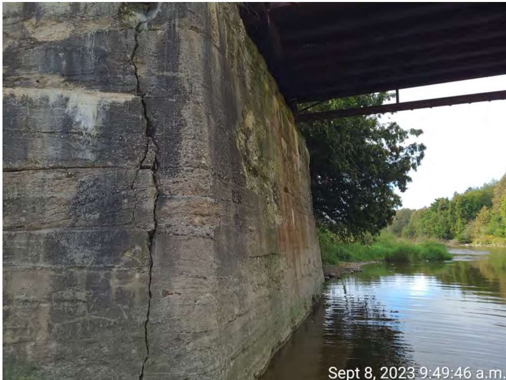
Photograph 18: East abutment, north wingwall showing wide vertical crack at wingwall/abutment interface. Footing repair visible below waterline.
