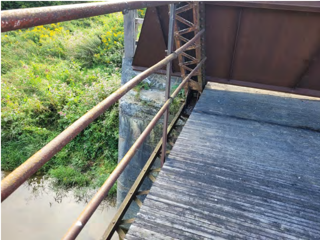
Photograph 1: Deck at east abutment, north truss. Note weathering of deck and triangular daylight below steel barricade wall indicating settlement of deck towards north truss.
