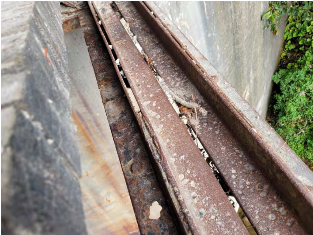
Photograph 14: North truss, Bay 9 bottom chord showing previous repair of angles welded between original bottom chord angles and lacing bars (date of repair unknown).
