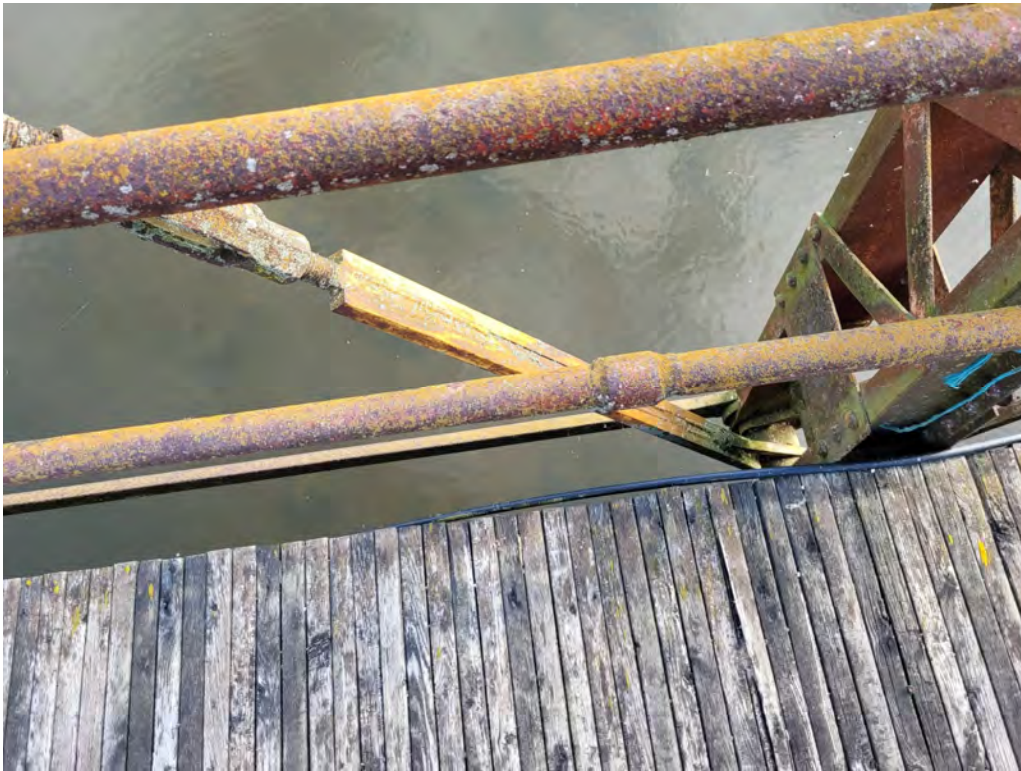
Photograph 13: North truss, Bay 4 counter diagonal showing previous repair of square bars welded to eye bar (date of repair unknown).
