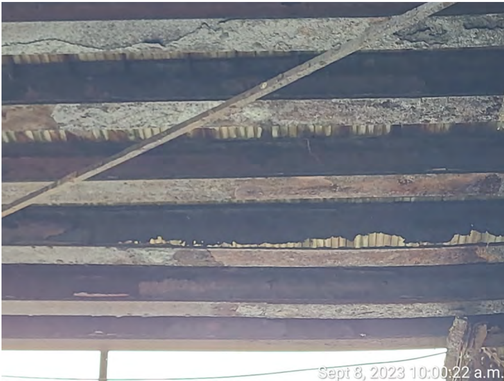
Photograph 4: Stringers in Bay 1 looking north. Note complete loss of section in stringer webs.
